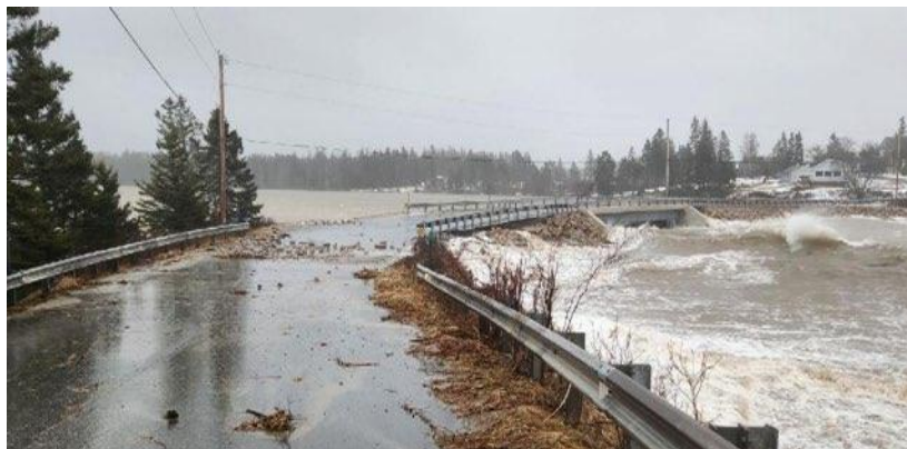
2 Johnson Cove Rd bridge overtopped during coastal storm, December 2023
